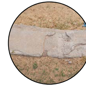
missing and cracked concrete
