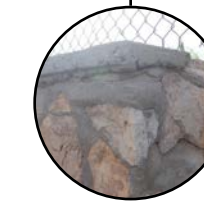
incompatible patching materials (mortar)
