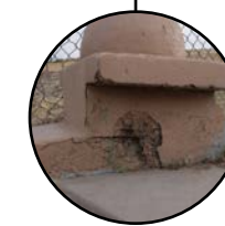
spalling due to corroded rebar
