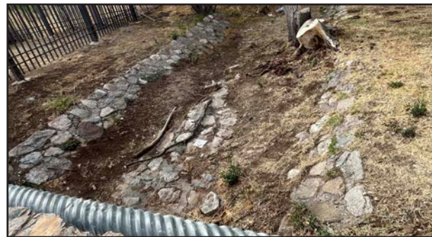
Debris and pipe in culvert bridge
