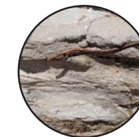
corrosion in exposed rebar
