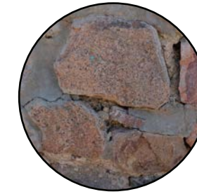
incompatible patches and failing mortar
