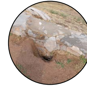
vermin infestation (holes under masonry)
