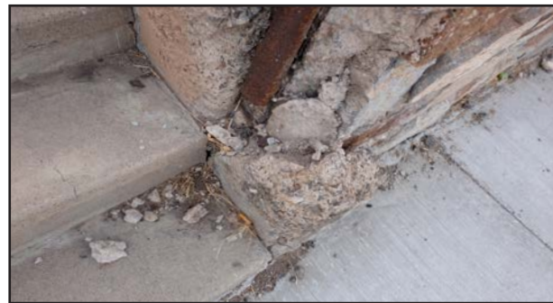
Typical interior structural failure
