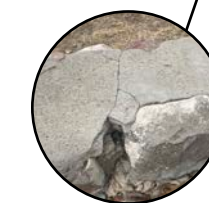
cracking and missing material (concrete)
