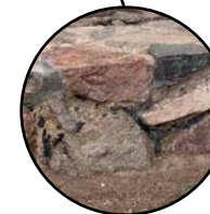
missing and loose material (mortar)
