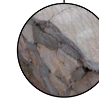
broken coping (concrete)
