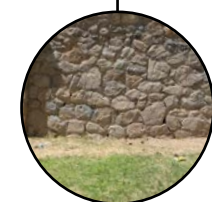
step crack (stone)
