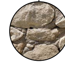
missing and cracked mortar
