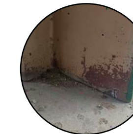
paint loss, cracks, and chipping (concrete)
