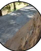
incised graffiti (concrete)
