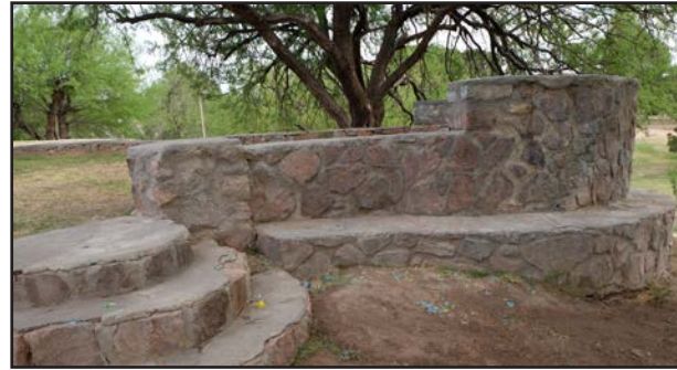
Erosion at rear of bench structure
