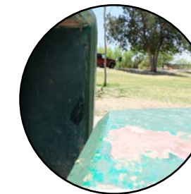
peeling paint (concrete)
