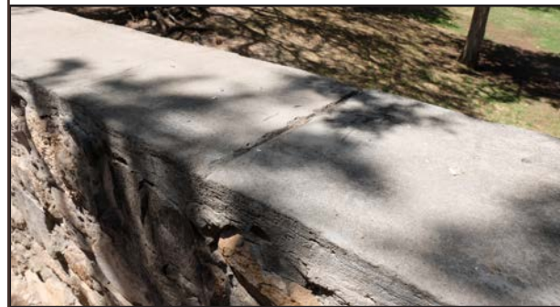
Scoring on concrete at top of walls
