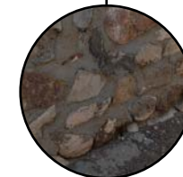
missing material (mortar)
