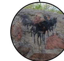
applied graffiti (paint on concrete)
