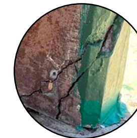
dislodged fragments (concrete)
