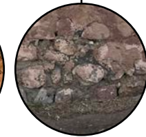
soiling and missing mortar near foundation
