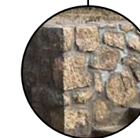
incompatible repair (mortar)
