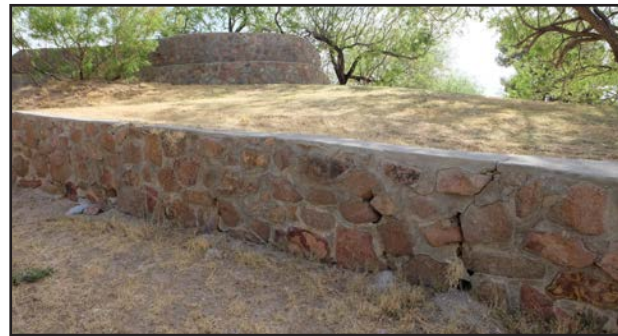
Step cracks from differential settlement
