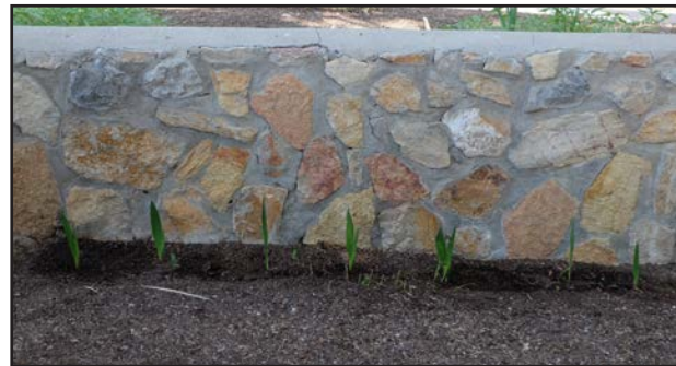
The interior rose garden walls are in good condition with some cracks in the concrete coping.
