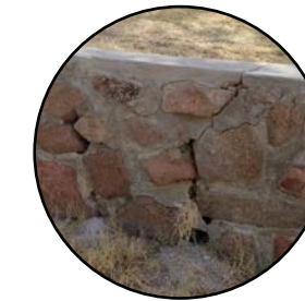
step cracks from settlement
