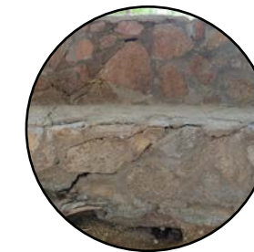
settlement from erosion
