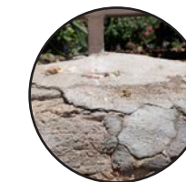
incompatible repair (mortar)
