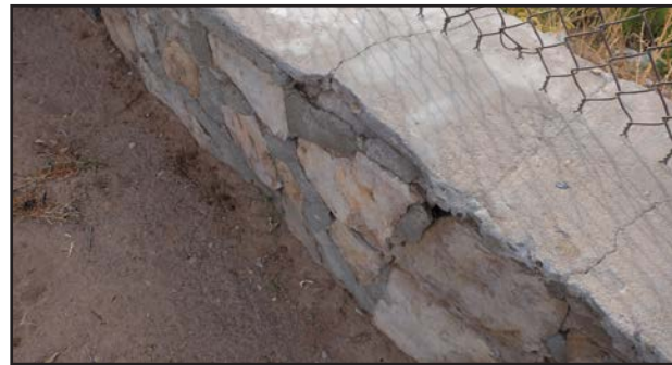
Scoring on concrete at top of walls
