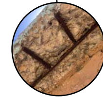
corrosion (structural metal)
