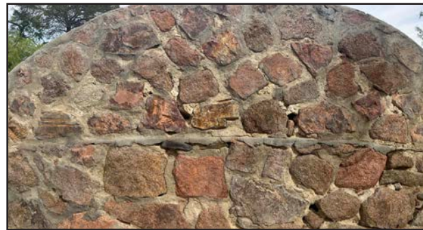
Missing mortar on rear of bench
