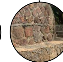
missing and loose material (mortar)
