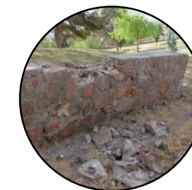
mechanical damage from human interaction
