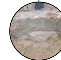
incompatible repair (concrete patch on stone)
