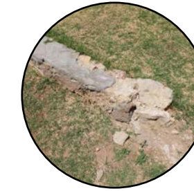
cracked, broken, missing sections of masonry
