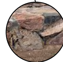
missing and loose material (mortar)
