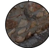
missing material (mortar)
