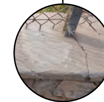
cracks in coping, especially where fence is attached (concrete)
