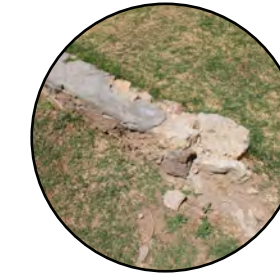
cracked, broken, missing sections of masonry
