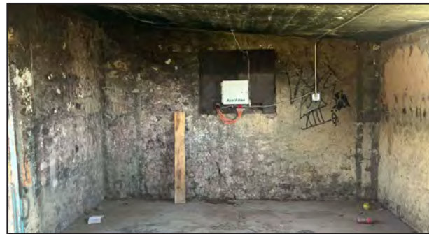
Accessory building interior with applied graffiti and deterioration
