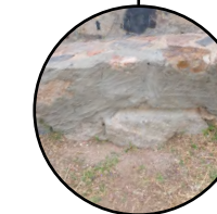
incompatible repair (concrete patch on stone)
