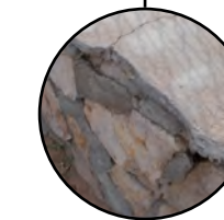
broken coping (concrete)
