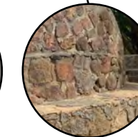
missing and loose material (mortar)
