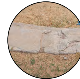
missing and cracked concrete
