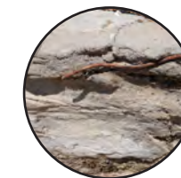
corrosion in exposed rebar
