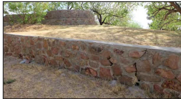
Step cracks from differential settlement
