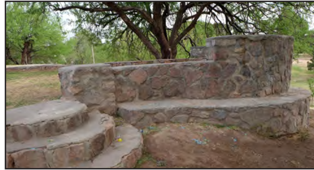
Erosion at rear of bench structure
