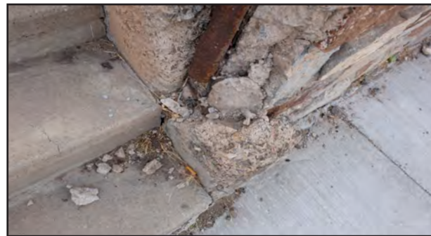
Typical interior structural failure
