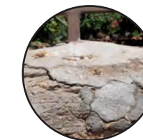
incompatible repair (mortar)
