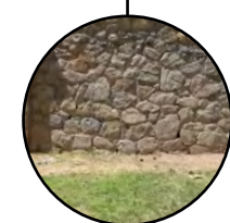
step crack (stone)
