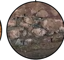
soiling and missing mortar near foundation
