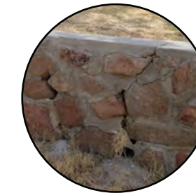
step cracks from settlement
