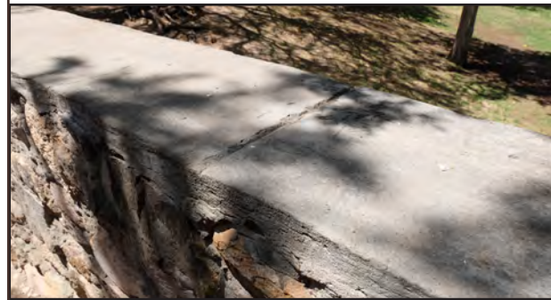
Scoring on concrete at top of walls
