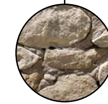
missing and cracked mortar
