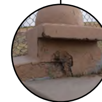
spalling due to corroded rebar
