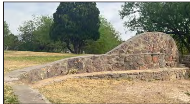
Back of bench; the adjacent ground should be monitored for erosion
