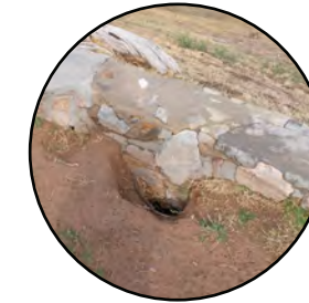
vermin infestation (holes under masonry)
