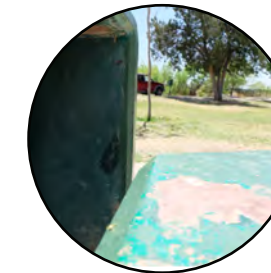
peeling paint (concrete)
