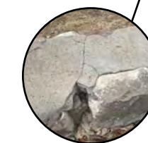
cracking and missing material (concrete)
