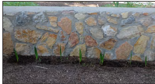
The interior rose garden walls are in good condition with some cracks in the concrete coping.
