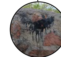
applied graffiti (paint on concrete)
