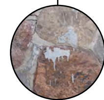
applied paint (masonry)
