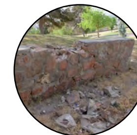
mechanical damage from human interaction
