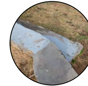
non-historic paint coatings
