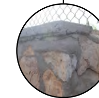
incompatible patching materials (mortar)
