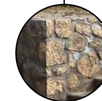
incompatible repair (mortar)
