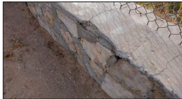
Scoring on concrete at top of walls
