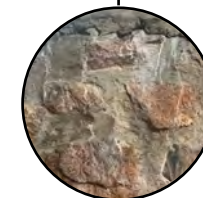
incompatible repair (concrete patch on stone)
