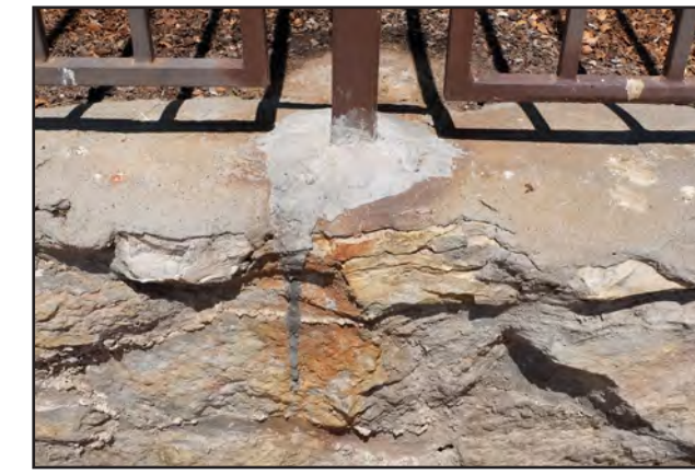
Incompatible repair patch, corrosion, and staining at the Rose Garden.
