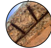
corrosion (structural metal)
