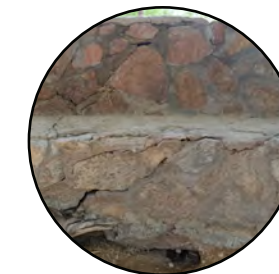
settlement from erosion
