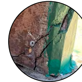
dislodged fragments (concrete)
