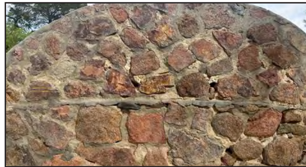
Missing mortar on rear of bench
