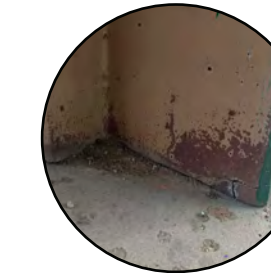
paint loss, cracks, and chipping (concrete)
