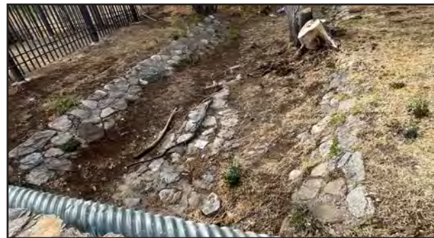
Debris and pipe in culvert bridge
